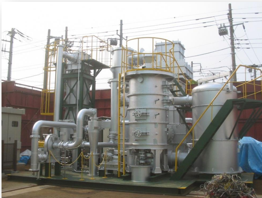
Our pyrolysis reactor as production unit
